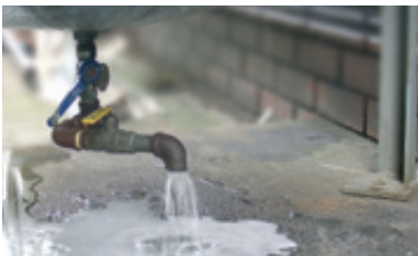
Contaminant Source No. 4 The Distribution Piping
