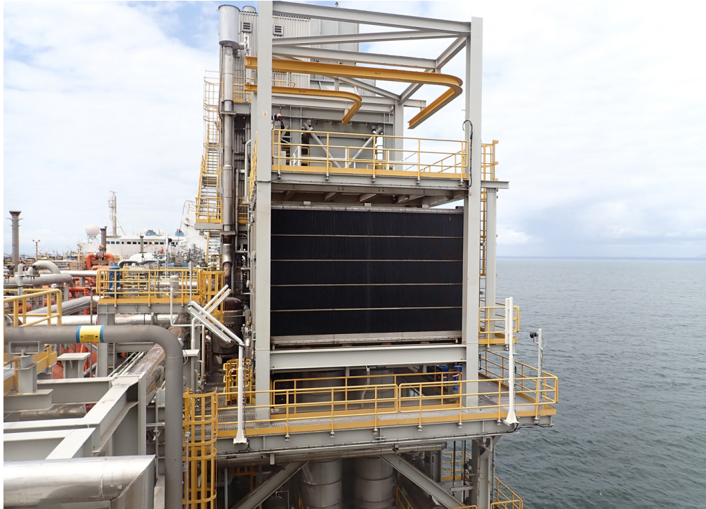
Fig. 2. Golar Hilli Episeyo's gas turbine (GT) air intake/filtration system (4 x PGT25+G4 GTs).
