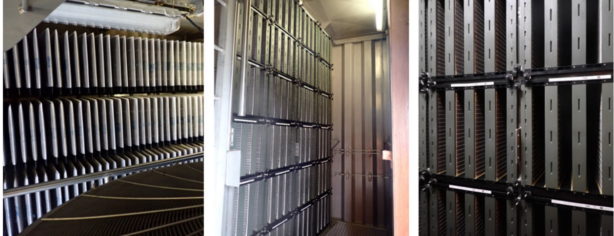
Fig. 4. View inside a high velocity GT filterhouse on the Golar Hilli Episeyo FLNG vessel. Left: The M6 rated prefilter. Centre and right: The E12 rated hydrophobic final filter.
