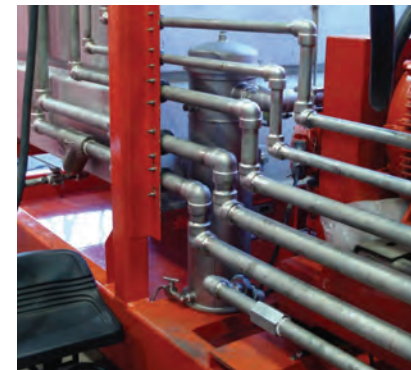
Figure 2 – Piping system with socket weld elbows and tees.
