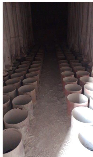
Thimbles welded to the tubesheet invite dust collection and corrosion.
