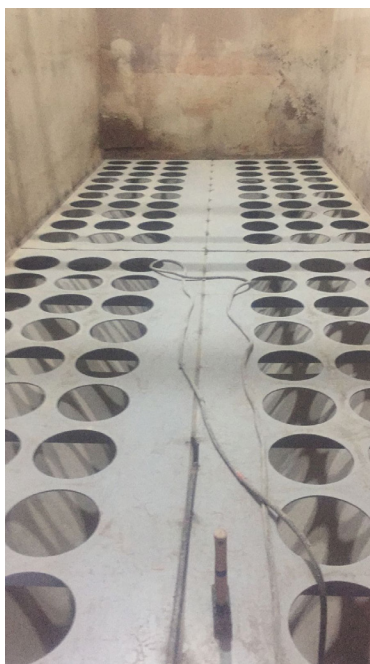
The custom tubesheet's flush surface allows quick broom clean-up.
